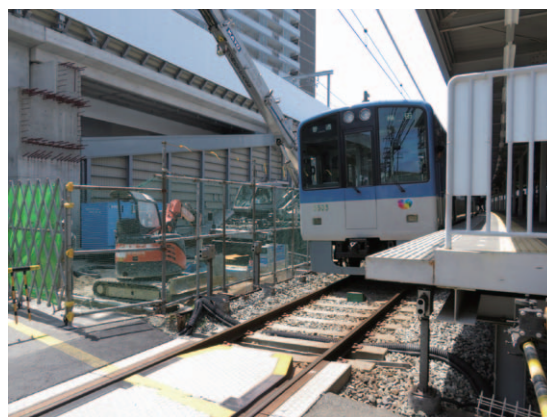
Construction work on elevating the platform at Fukae Station of Hanshin Railways is underway, using a method that ensures the groundwater is protected (Higashinada Ward, Kobe)
